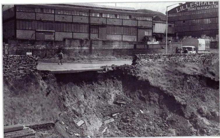
George Nock, Bill Tranter, and Clifford Briggs, all of Ketley Bank, were walking down the A5 from the Lilleshall Company on Sunday, May 22, 1966, when they noticed a hole in the parapet, and then saw that a bank had subsided. As they directed traffic to the other side of the road, the parapet collapsed. The landslide closed Shropshire's main traffic artery, the A5, at Oakengates. A railway bridge by the Greyhound crossroads partly collapsed, demolishing part of a parapet and the footpath. The bridge took traffic over the disused Wellington to Coalport railway line and carried gas, water, and sewerage mains.
